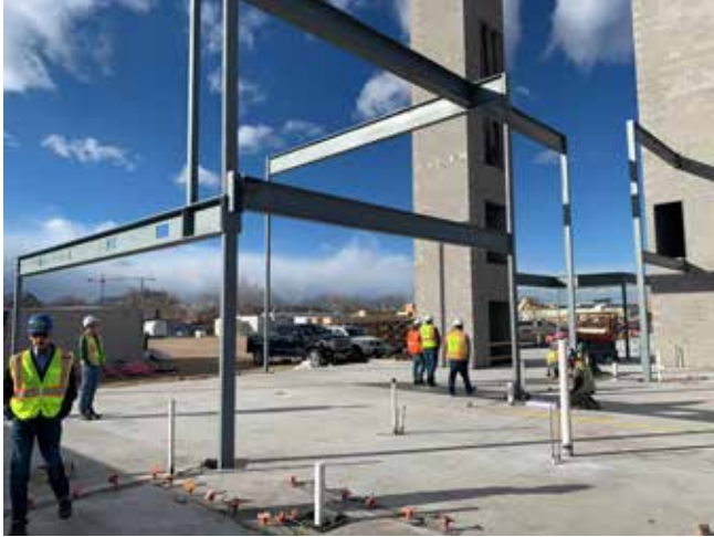
Image: Courtesy of Mile High Ministries Construction workers in December 2022 work in northern Denver at the site of the future Clara Brown Commons apartment building. Mile High Ministries, a faith-based organization that has served low-income people in the Denver Metro area for more than 30 years, is developing the property.
